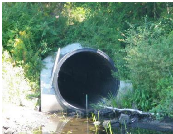
This "perched" culvert requires a swimming or leaping ability that not all fish or wildlife have.
